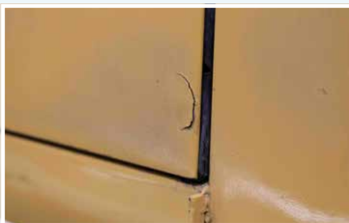
Splits, cracks in paint often reveal a multitude of sins
